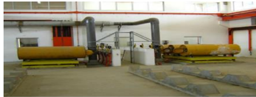
CHLORINE SCRUBBER SYSTEM
